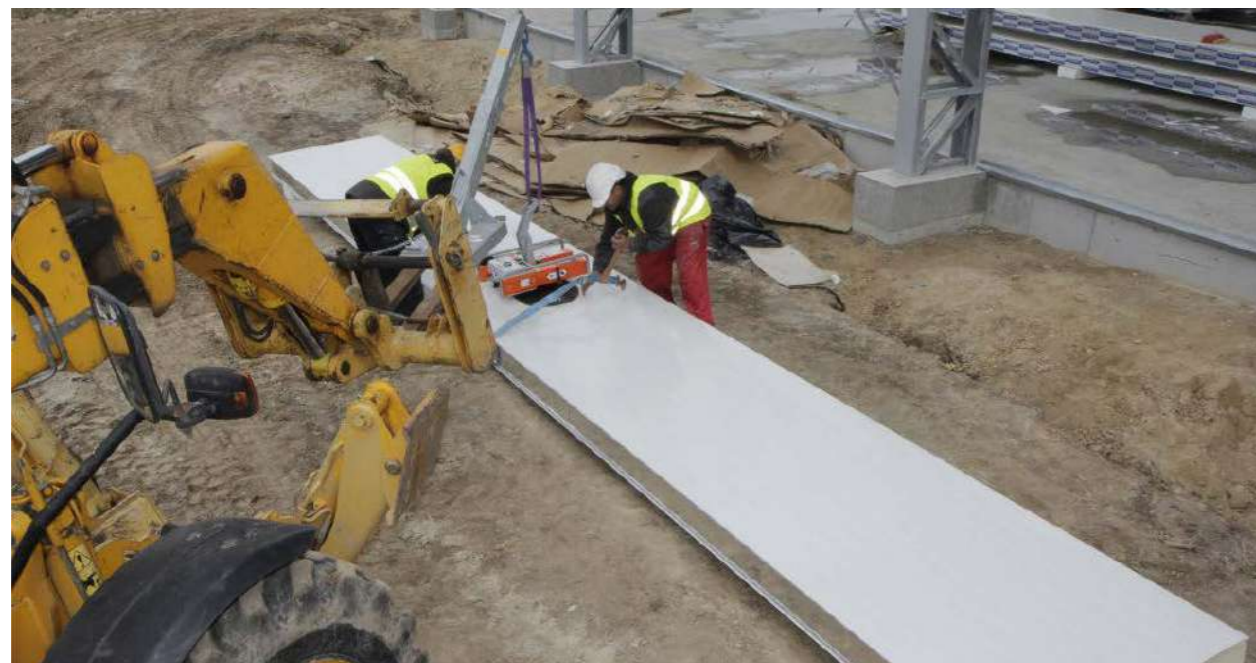
Photo 8. Lifting a panel from a stack using a vacuum suction cup (horizontal installation).
