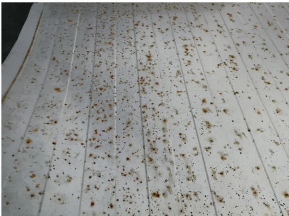
03. Advanced pitting corrosion
